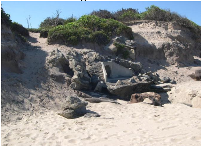
One of the outlets causing serious erosion along the Lake Cathie beach south of the entrance
